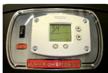
Honeywell control panel
