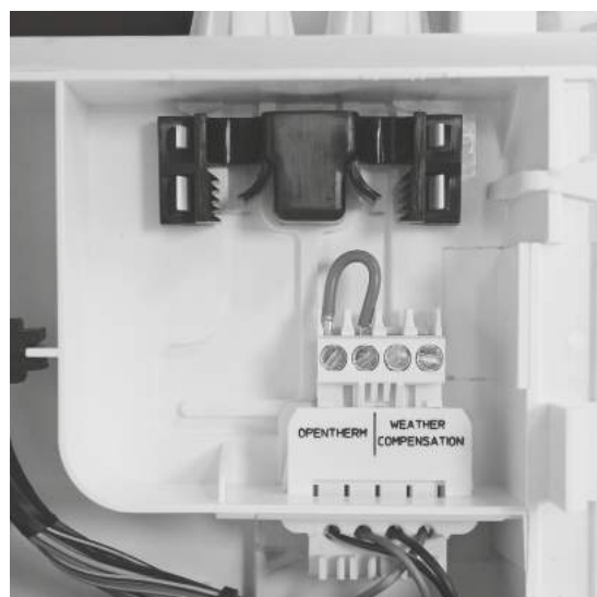
INSTALLER CONNECTIONS (RHS)
