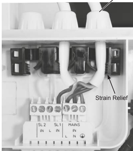
INSTALLER CONNECTIONS (LHS)
