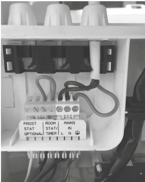
INSTALLER CONNECTIONS (LHS)
