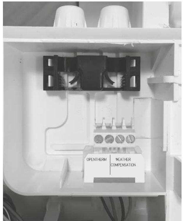
INSTALLER CONNECTIONS (RHS)
