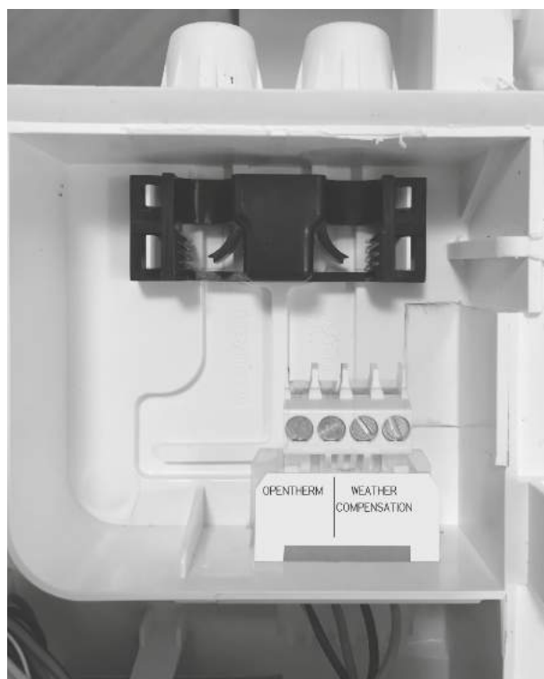
INSTALLER CONNECTIONS (RHS)
