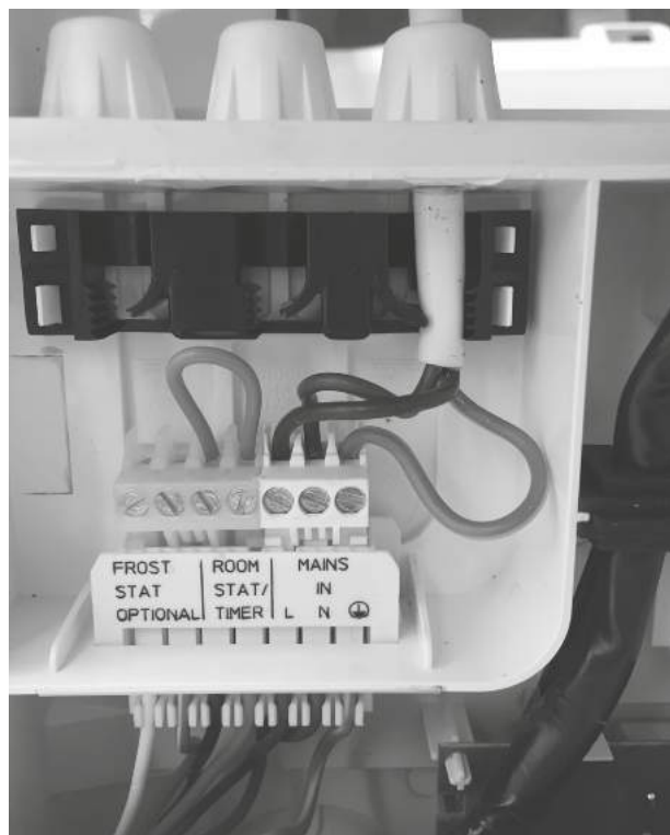
INSTALLER CONNECTIONS (LHS)
